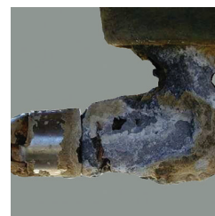
Unprotected sail drive
